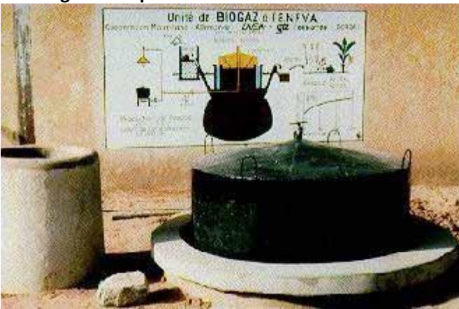
Figure 7: Floating-drum plant in Mauretania
